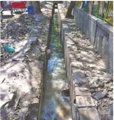
Condition of Stormwater Drain
