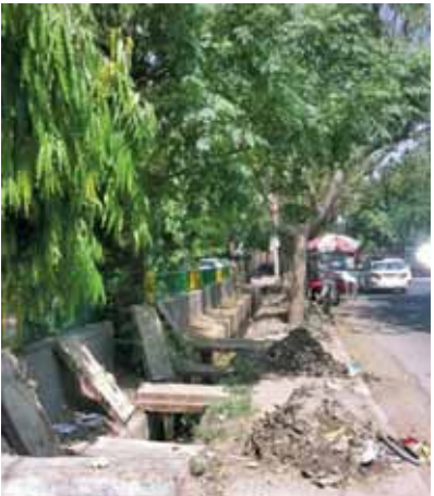
Clogged Stormwater Drain
