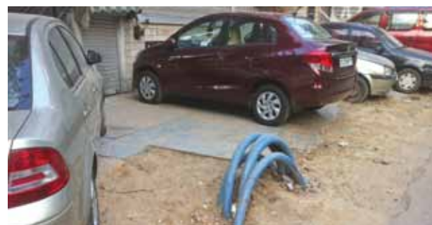
Cables protruding from Ground
