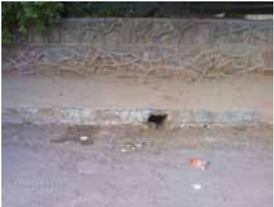
Condition of Stormwater Drain
