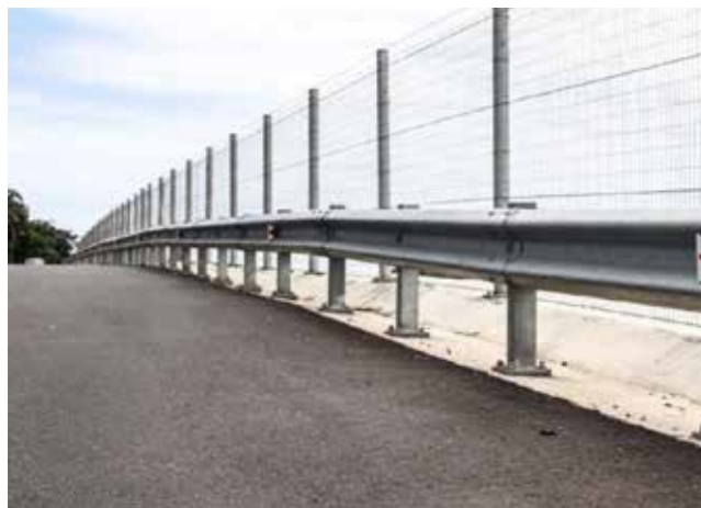
Guardrails obstructing the crosswalk
