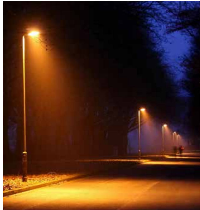
Street lighting inappropriately placed, leading to dark patches in between that render the street unsafe for pedestrians
